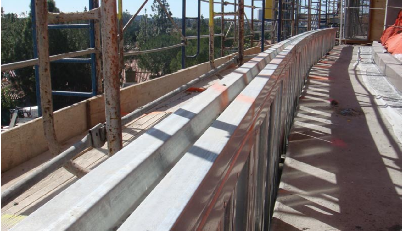
A three-piece unit for this exterior radius was constructed to replace the 12-piece assembly that was originally specified for the building. This significantly reduced labor on the jobsite.
